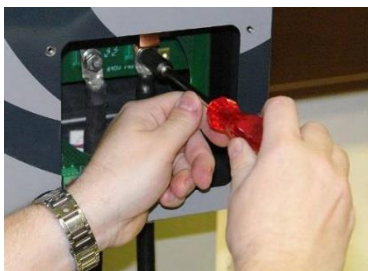
Fig. 13: Connection track cable (with unmounted cover plate)
